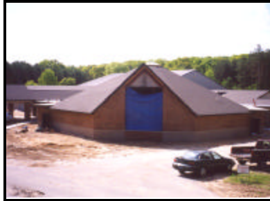
Top: Ross Bible Church as the finishing exterior details are applied Bottom: Lakeshore Baptist Church during construction
