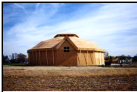
Above: Farmland Friend's 110' geodesic dome after assembly. The Farmland, Indiana, congregation chose an 18' sidewall with the gable option.
