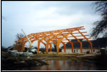
Above: Setting arches for Christian Love Fellowship's rectangle structure in Ypsilanti, Michigan.
